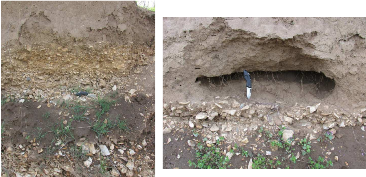
Figure 42. Streambank at the Barren Fork Creek field site including the bank profile (left) and a seepage undercut (right). Note the sloughed material in the bottom of each picture from recent bank failures. These complex alluvial deposits include both clean gravel lenses associated with rapid flow and transport (left) as well as fine gravel lenses that can cause lateral flow and seepage erosion.
